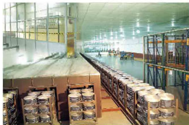
隧道窑 Tunnel Kiln
